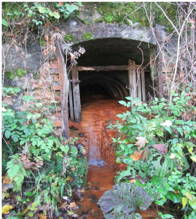
Figure 1: Discharge of mine water from the Sava tunnel with the disposal of mine sludge
