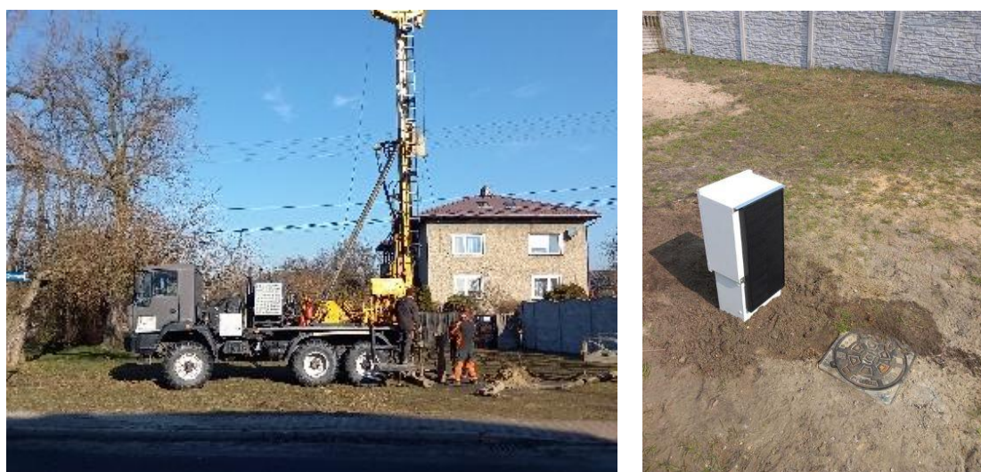
Figure 5. Photos documenting the installation of the TRZEBINIA2 automatic hydrogeological station at the Siersza test site of the SIRIMA project.
